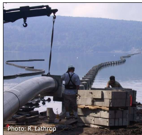
Figure 17. Installation of the siphon pipe in Devils Lake in August 2002. Source: 14 Lathrop 2021
